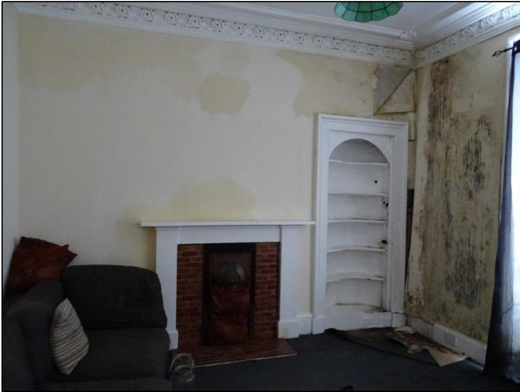
Photograph showing the interior of 106 Flat 1 taken in January 2020 showing the level of water ingress and rot
